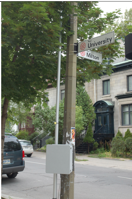
E: Installed Enclosure And Deployed Mast As Seen To Pedestrians. Power System Is Inside Enclosure
